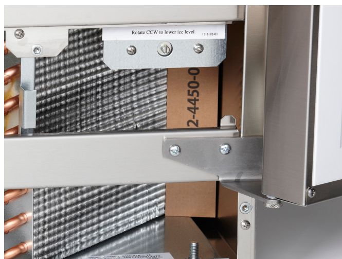
Condenser and Bin Thermostat
